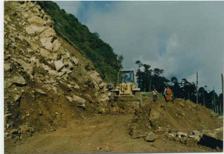
Figure 17: Pay Loader clearing landslide
