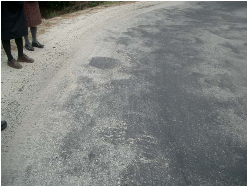
Figure 10: Flushing/Bleeding and shoving
