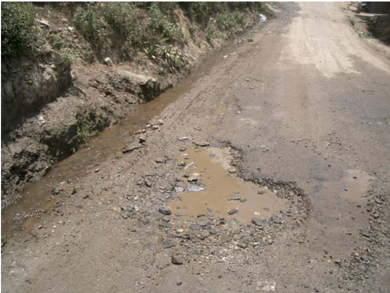
Figure 6: Pothole created by seepage of drain water
