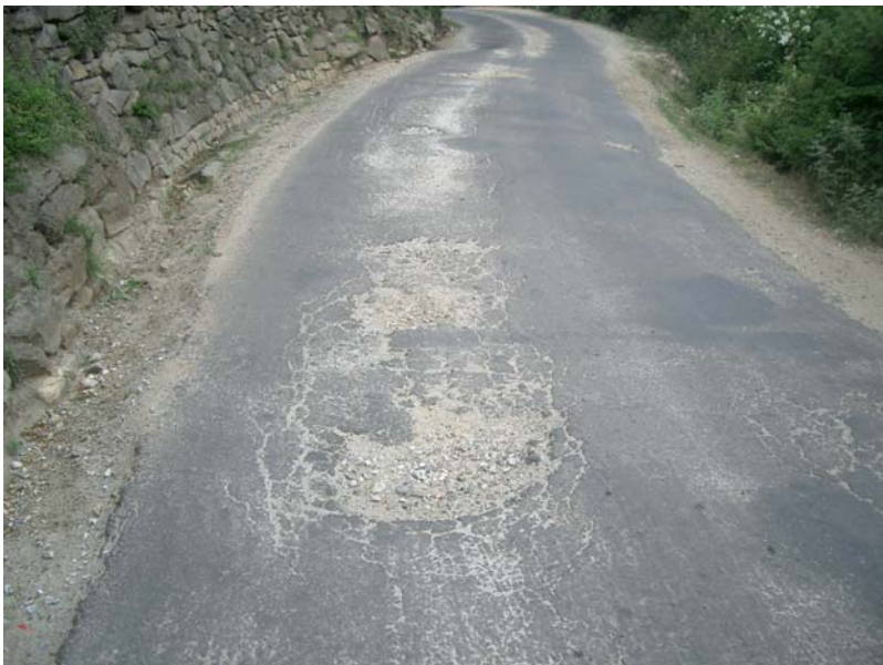
Figure 8: Pothole and Longitudinal Cracks
