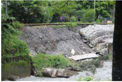
Figure 2: Damages caused by Dhoti Khola.
