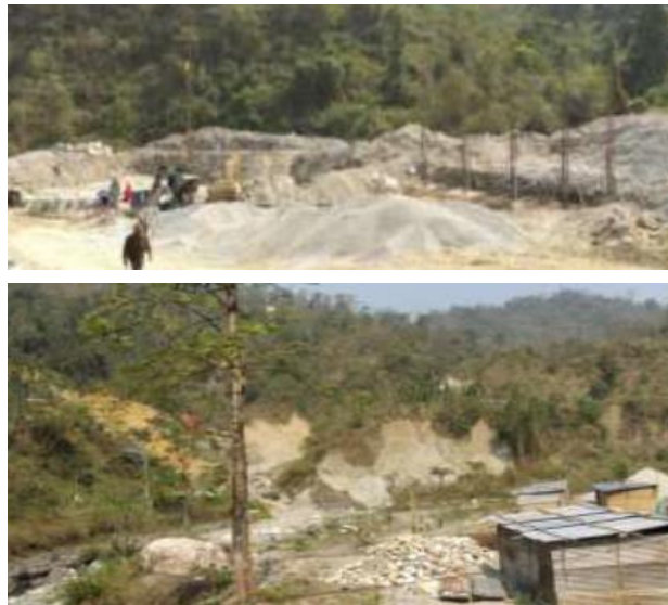
Figure 22: Construction on the left bank of a tributary of Dhoti Chhu (River).
