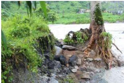
Figure 5: River bank erosion during the flooding.
