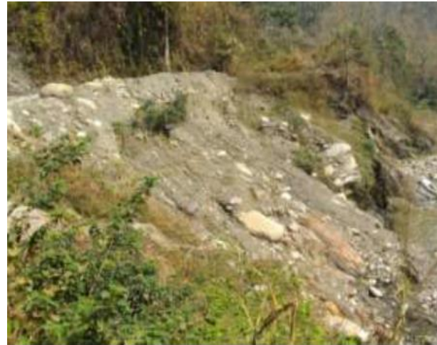
Figure 24: Erosion at the road base by Barsa chu above BPC sub-station at Pasakha.
