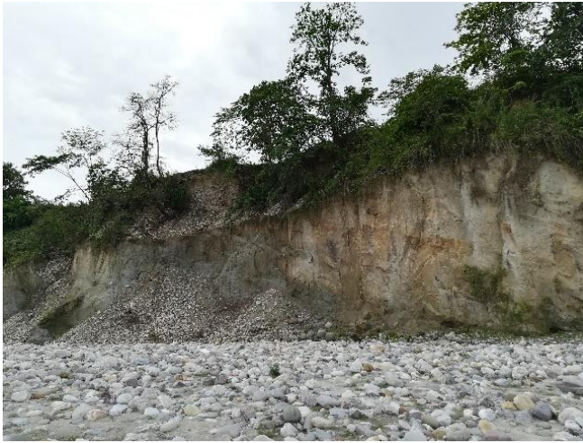
Figure 15: Scouring at the base of Hawajorey village by Sunkosh river
