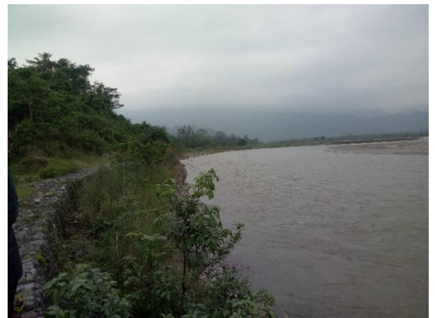
Figure 18: Scouring/Erosion by Sunkosh River in Majagoan village
