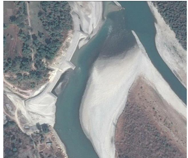
Figure 30: Sunkosh River in 2017 after the construction of gabion revetment and spur at the right bank of the river.
