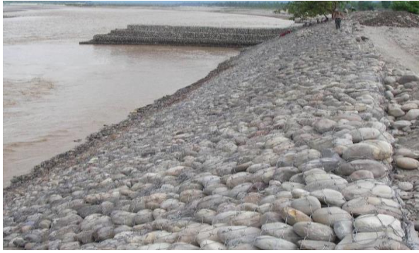
Figure 24: : A typical combination of revetment and spur, Mahakali river, Nepal
