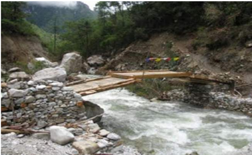
Figure 16 wooden bridges washed away by the rivers during monsoon rain.
