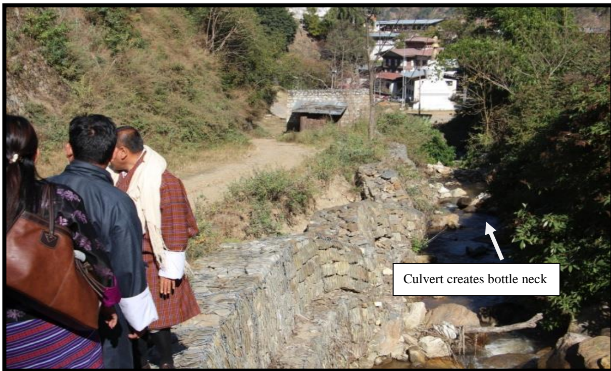
Figure 11: Culvert create bottle neck during heavy monsoon season and not able to accumulate whole discharge.
