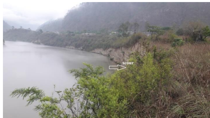
Figure 15: Location of scouring area in Gyalposhing.
