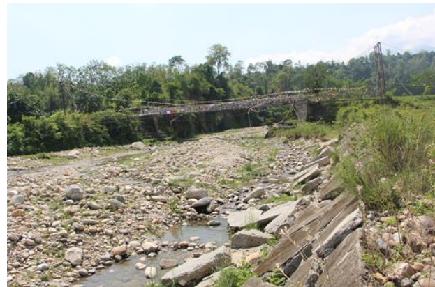
Figure 8: Existing RRC revetment was destroyed in 2016 flooding.
