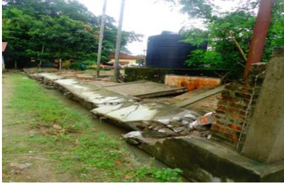
Figure 2: Compound wall damaged.
