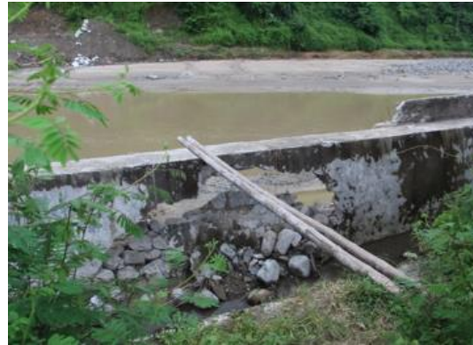
Figure 5: Flood protection structure damaged.
