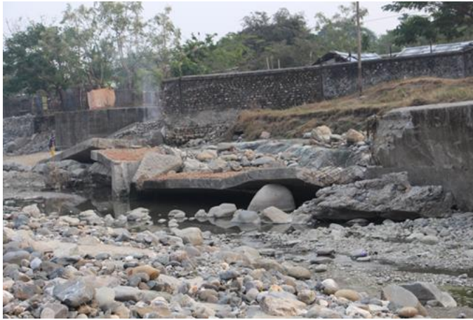
Figure 17: Damaged wall near international border
