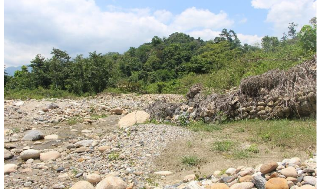
Figure 11: Existing Gabion wall has failed.
