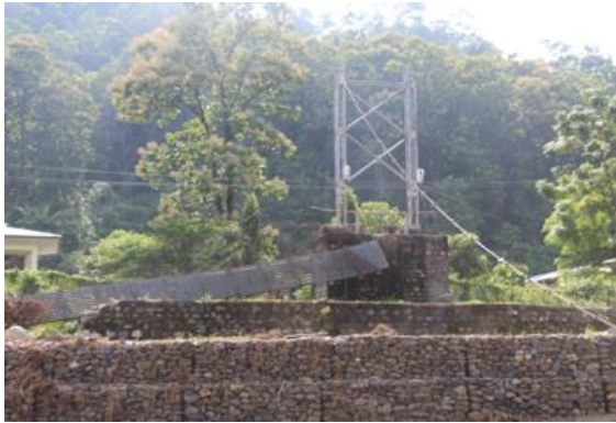
Figure 4: Suspension bridge damaged.
