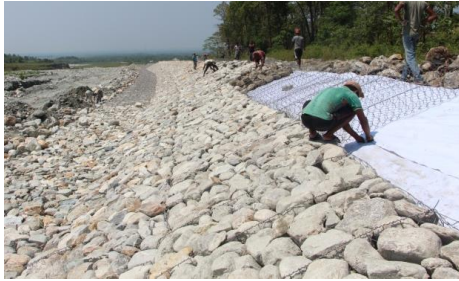
Figure 11: gabion revetment along right bank of Sukriti River during construction in June, 2017.
