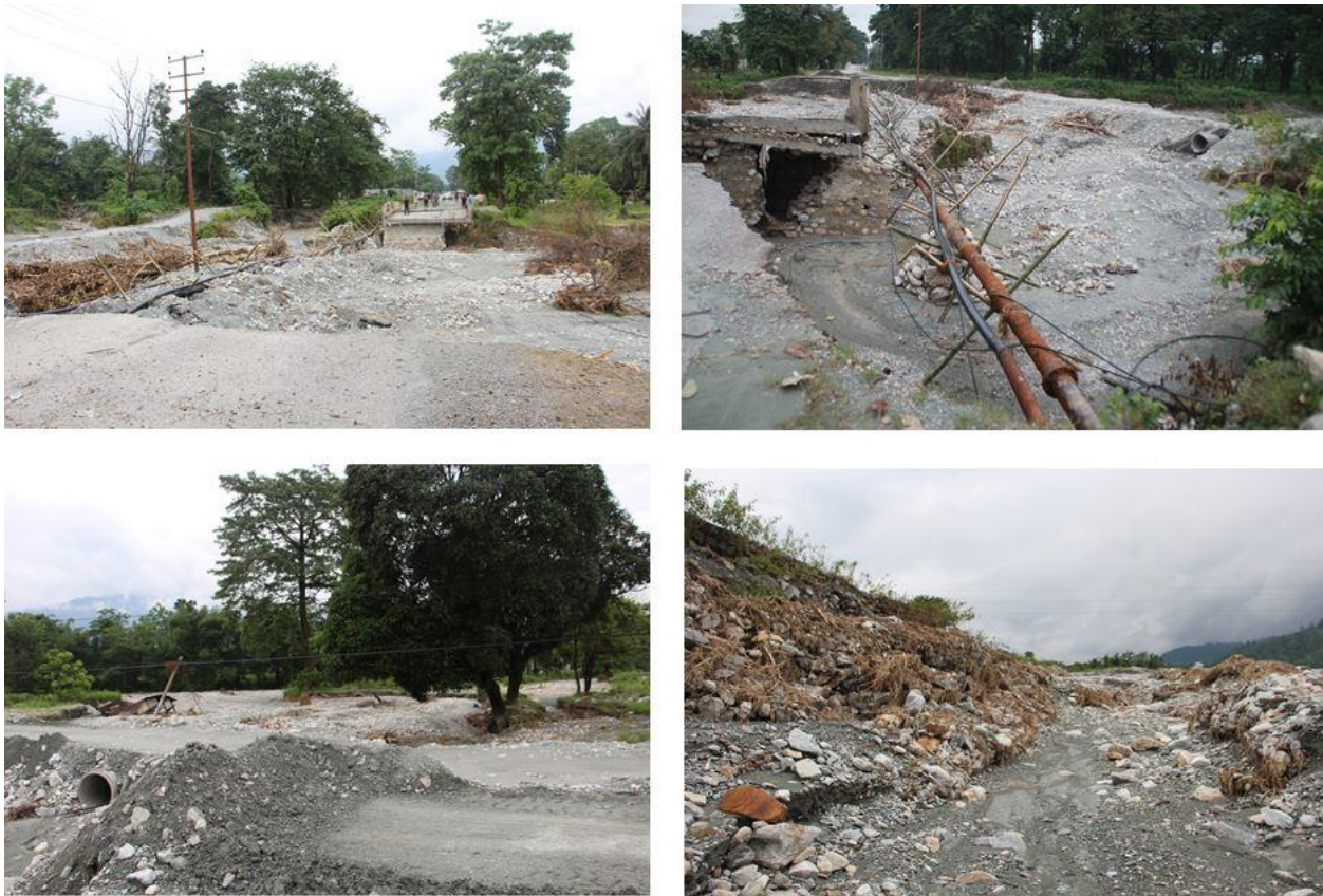
Figure 29: Destructions caused by the Shetikheri stream.
