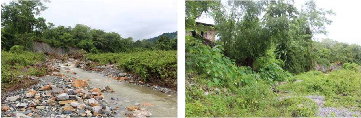
Figure 32: Minor landslide and scouring along Jangkukung chu.
