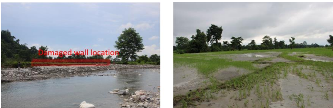
Figure 30: Damaged wall and affected paddy field locations.
