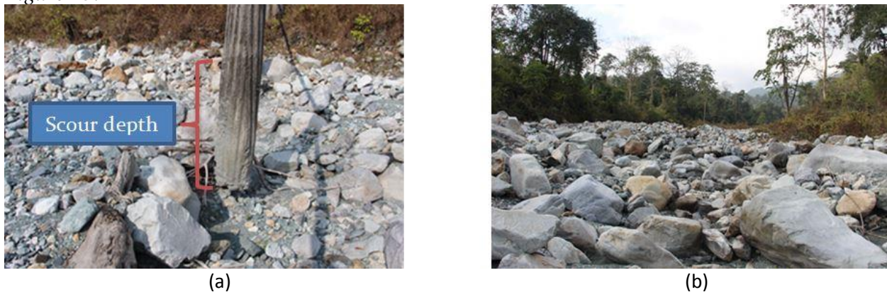
Figure 15: (a) Scour depth on the pillars (b) Debris collected at the downstream of Shetikheri.
