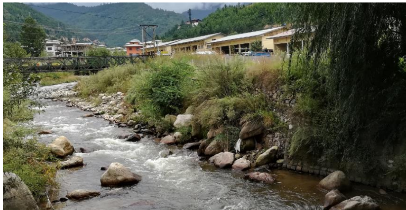
Figure 37: Exposed workshop area without gabion wall protection
