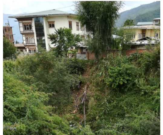
Figure 31: Need for slope stabilization below RENEW office.
