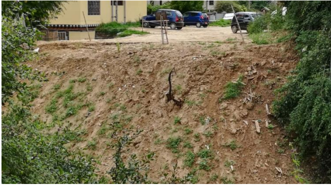
Figure 30: Need for slope stabilization downstream of ELC school.
