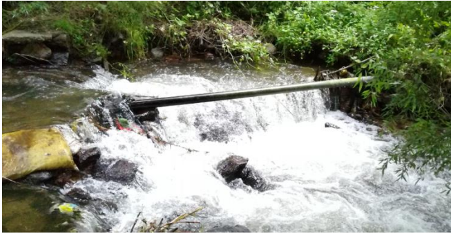
Figure 28: A water supply pipe running across the stream upstream of Desi Zam.
