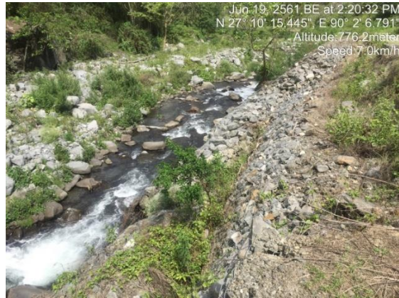
Figure 5: Failure of Gabion wall constructed by PHPA II along Kamichu
