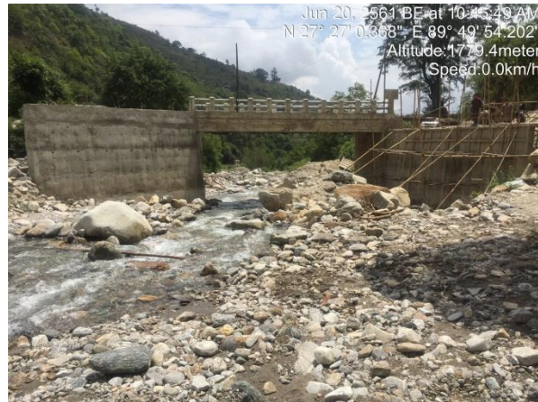
Figure 18: Bridge connecting Yusawom and Yusagom Chiwang is under reconstruction after it was washed away in 2016
