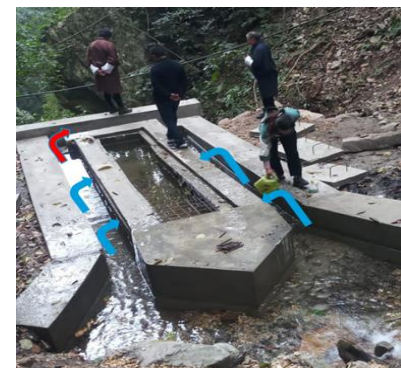
Pic-6: RCC filtration intake structure is a climate resilient technique to secure quality of drinking water
