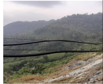
Pic-3: Avoiding landslide areas by crossing hung water pipes overhead. This measure will reduce recurrent repairs and maintenance cost and other resources such as time and labors.
